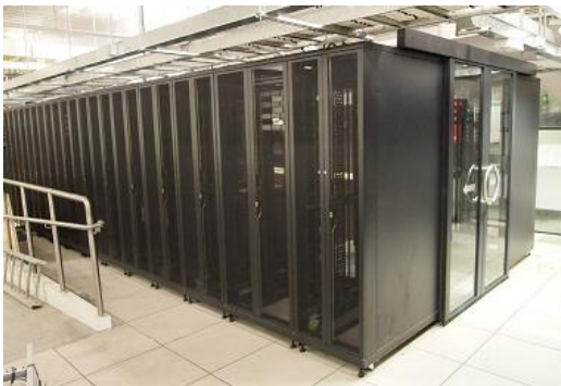
Example of Air-Trap Cold Aisle Containment System
